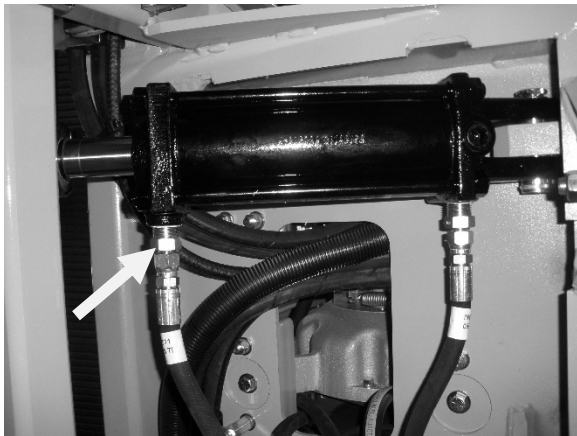
View showing left lift cylinder
